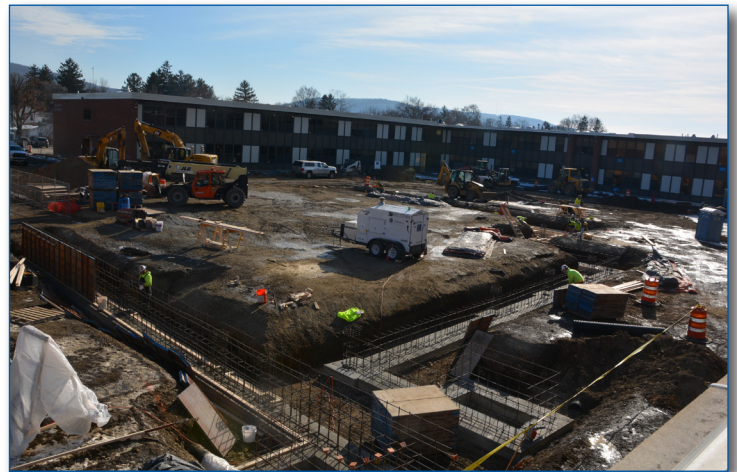
View of “the quad” at the High School, with construction of the new library and corridors to improve student traffic flow.
