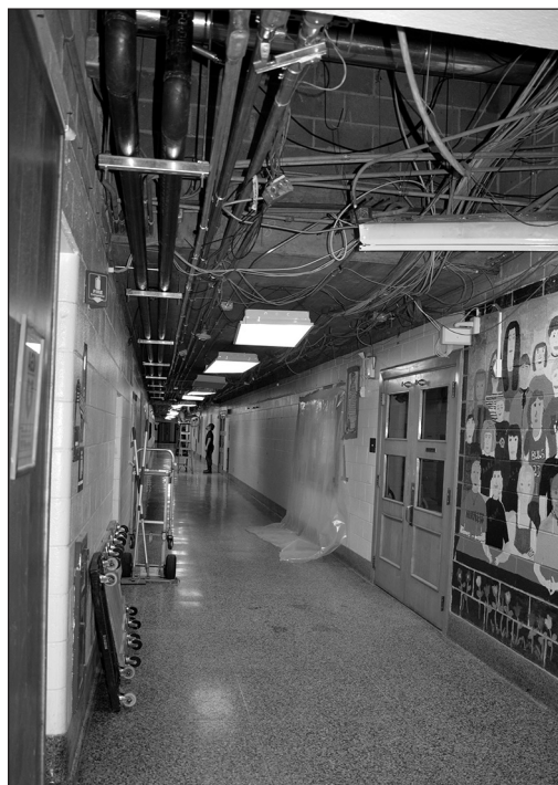
Portions of the ceiling at Ridge Road and all our elementary schools are being replaced to allow for new ductwork and other mechanical devices.
