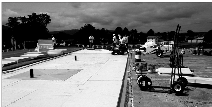
Portions of the roof at Big Flats have been replaced this summer.
