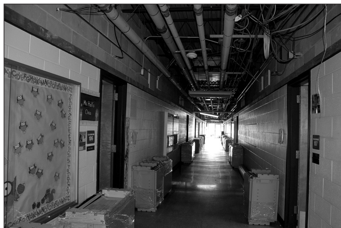
Gardner Road will have new heating/ventilation and ductwork. All corridor ceilings will be raised when reinstalled.
