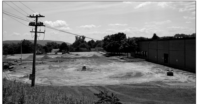
The parking lot at Gardner Road, which was at the end of its useful life, is being replaced and will create better traffic flow and a safer parking area for students, staff, and parents.
