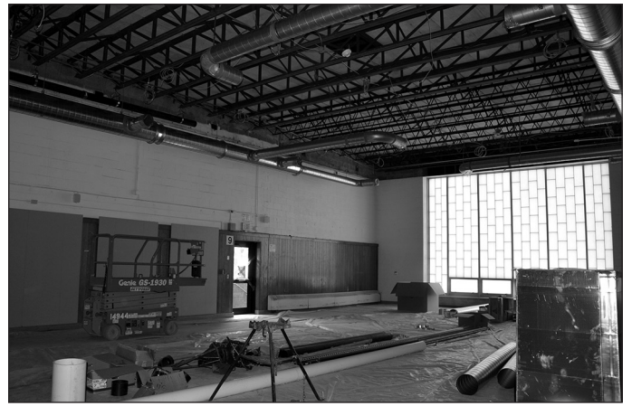
The ceiling at Center Street is removed in preparation for new ductwork and new roof drains.
